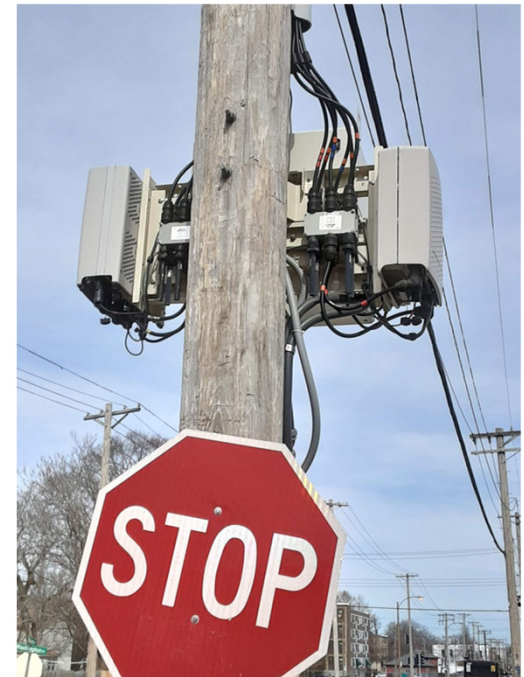
St. Louis, MO - Ameren Utility Pole
